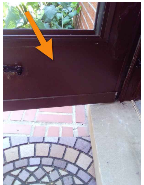
Missing pneumatic cylinder closing mechanism
