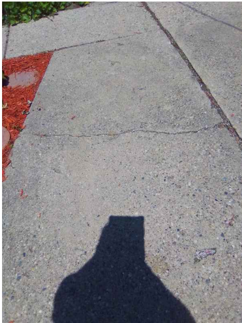
Simple cracks that can be easily filled in with a concrete tube
