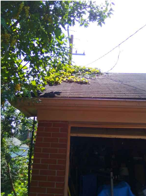
Over grown vegetation from neighbors yard.
