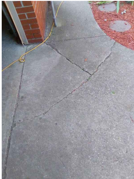
Simple cracks by entrance of garage they can easily be repaired with simple concrete caulking
