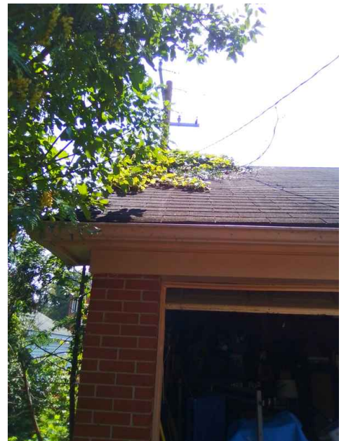
Over grown vegetation from neighbors yard.
