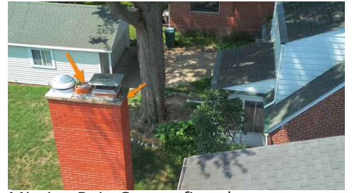
Missing Rain Cap on fire place stove exhaust. Should be properly covered. Recommend point and tuck mortar repair.
